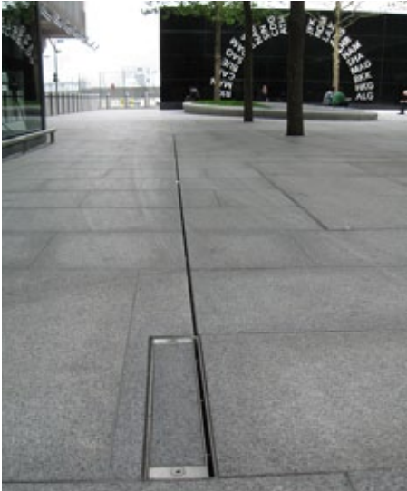
ACO Brickslot used in the ground floor plaza area
