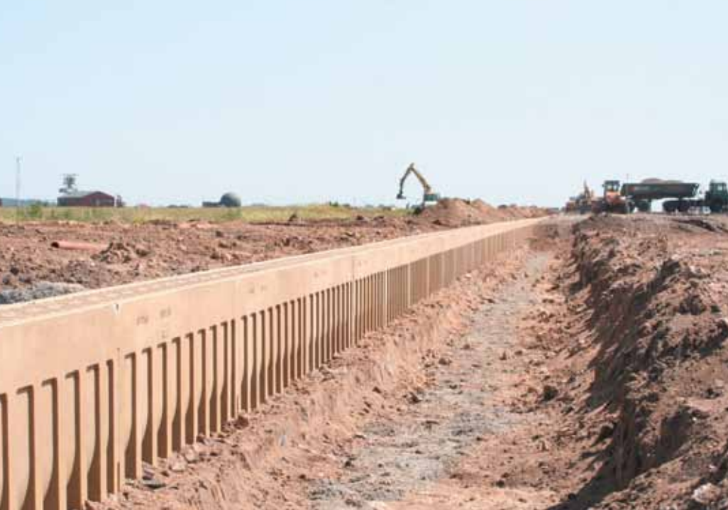
ACO DRAIN® Monoblock drainage channels along the take-off and landing runway
